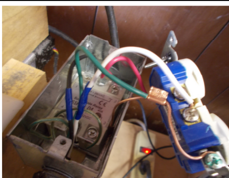
Figure 5. Solid state relay allows software control of the router.
