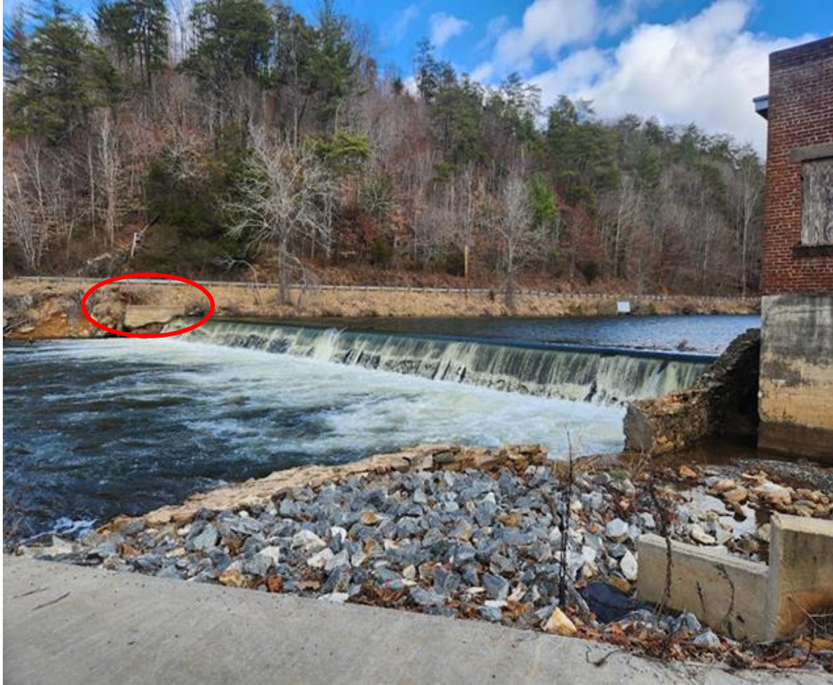
Figure 2. Cullowhee Dam 2023. The red oval indicates an area of the dam where water diverts around the dam during high-flow periods, undercutting the bank. Without repair, erosion will occur under the adjacent road.
