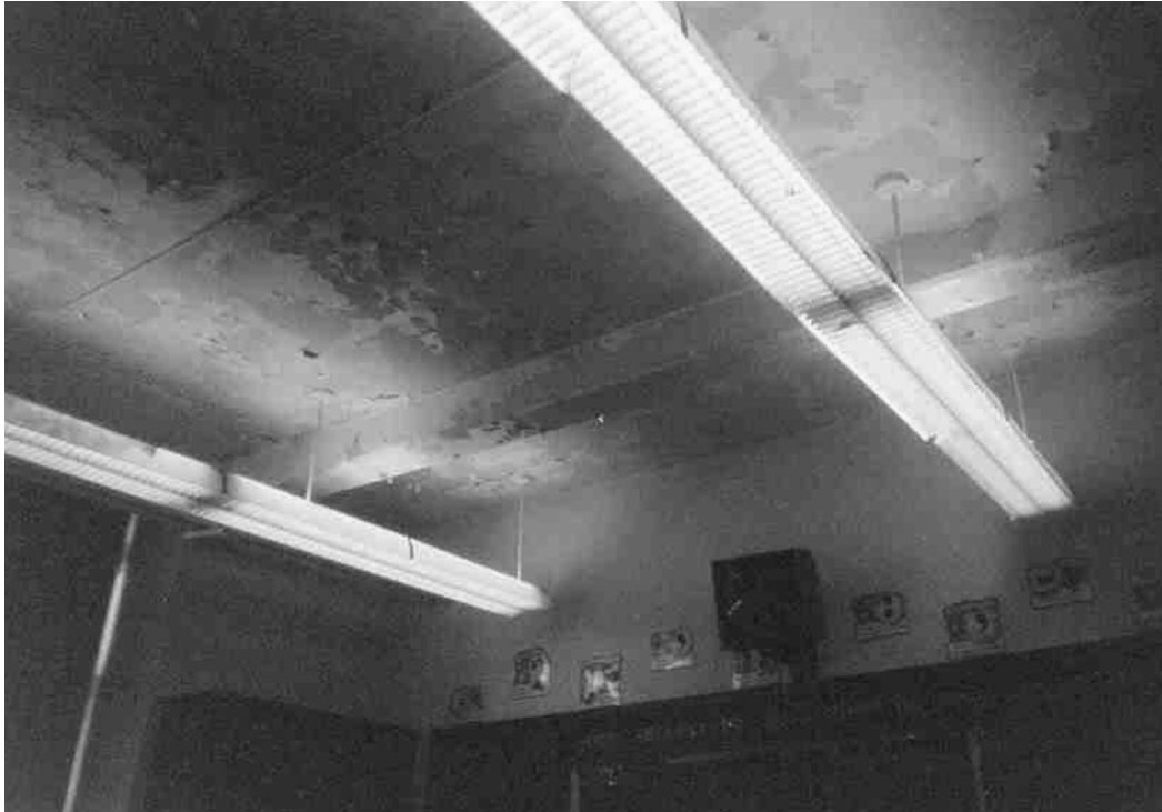
FIGURE 3 My middle school is a bad school. The ceiling is falling apart and it is not good. SOURCE: Youth photographer, age 12.
