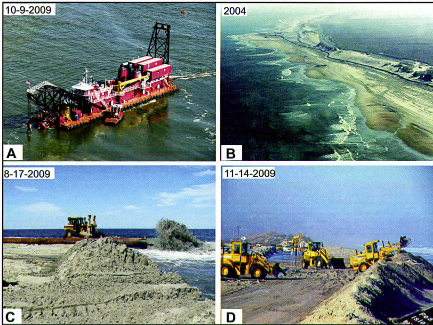
Figure 13. Figures show the Oregon Inlet dredging and beach nourishment in the Canal Hot Spot area of Pea Island. Panel A shows a pipeline dredge working in the navigational channel of Oregon Inlet. Panel B is an oblique aerial photograph showing a nourished beach being constructed. Notice NC Highway 12 adjacent to the beach in the upper right corner. Panel C shows a pipeline dredge delivering sand to the nourished beach. Panel D shows bulldozers constructing a new barrier dune ridge. All photographs are from the Pea Island National Wildlife Refuge.
