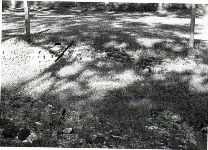
Figure 9. Photograph looking east along possible N60E-trending fault (black line) across the eastern wall of the powder magazine with the southern side (right) tilted downward. Small black rectangle is 15 by 20 cm notebook.
