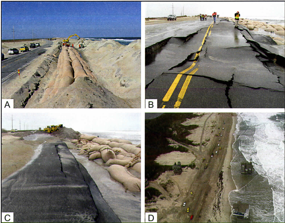
Figure 24. Ground and oblique aerial photographs of the S-Curves Hot Spot illustrate recent maintenance activity on NC Highway 12 in response to the Veteran’s Day Nor’easter of November 11, 2009. These photographs are at the same location as the red stars on Figure 23. Panel A shows the NCDOT construction of a sand-bag core for the barrier dune ridge in 2007. Panel B shows the destroyed sand-bag wall and NC Highway 12 (11-14-2009). Panel C shows the subsequent mining of the overwash sand and reconstruction of the barrier dune ridge on top of the broken sand bag wall (11-14-2009). Panel D is an oblique aerial photograph (11-19-2009) that shows the temporary vehicle by-pass while NCDOT relocates a portion of the road and reconstructs a new sand-bag-cored barrier dune ridge. Notice the two houses in north Rodanthe that are in the surf zone.
