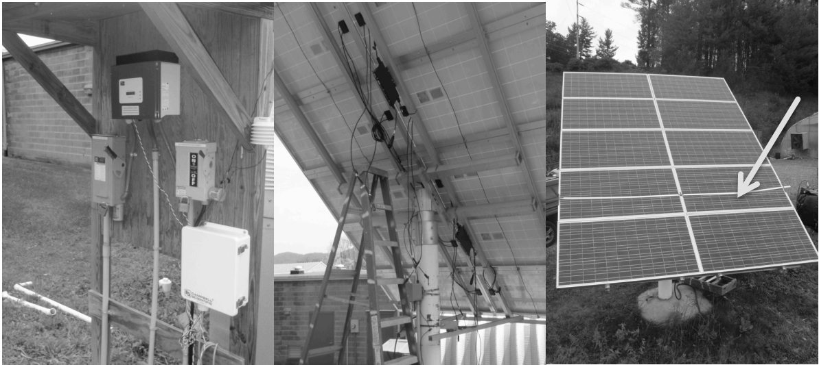
Figure 5. Photo of covered equipment mount area, with the SB700U central inverter, CR-800 data logger (white), and array disconnects.
